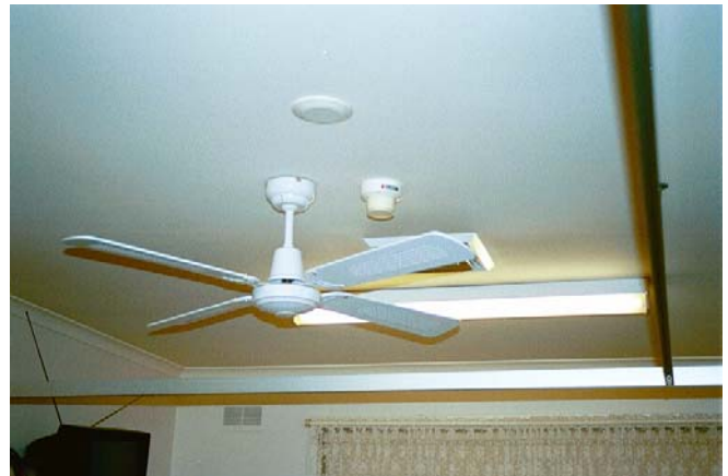
SMOKE DETECTOR WITHIN 400MM OF END OF FAN BLADE.
